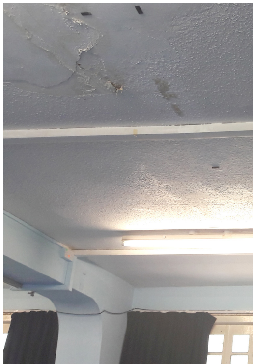
Water damage to existing ceilings
