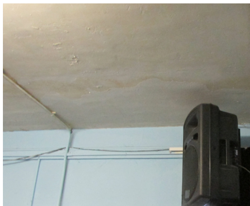
Water damage to existing ceilings
